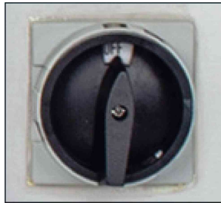
Power Switch shown in the "OFF" position
