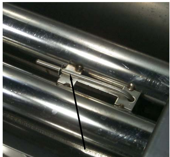
Electronic thermostat probe in frypot (arrow).
