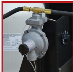
Regulator, Tee Check and Hoses
