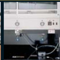
Hot Deli temperature controls and drains
