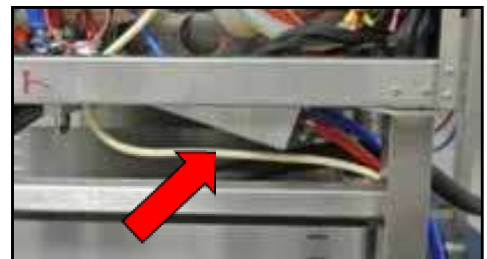
Delime hose underneath the oven.
