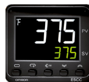
Electronic Controller located on door
